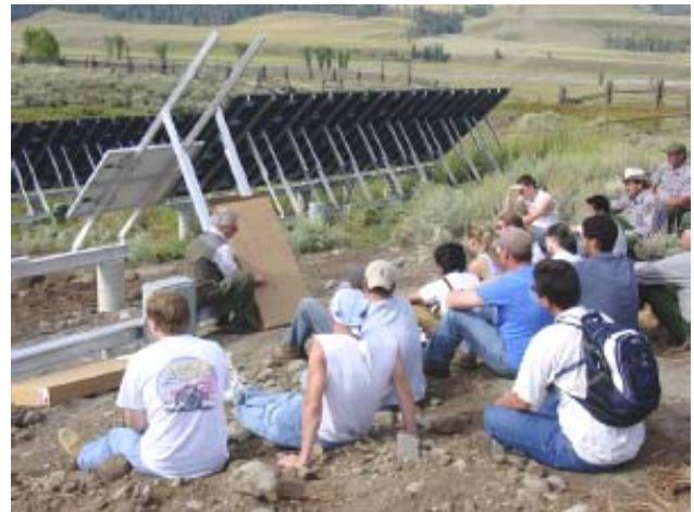
SDSU students and Yellowstone personnel (at right) learn about code-compliant PV installation
