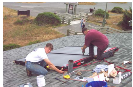
Kelly Miess and Andy Sorter install the solar thermal system at the Redwood National Park Kuchel Visitor Center.
