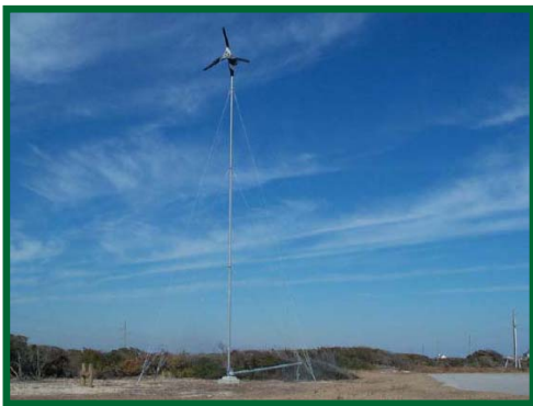
2.5kW wind turbine at Coquina Beach
